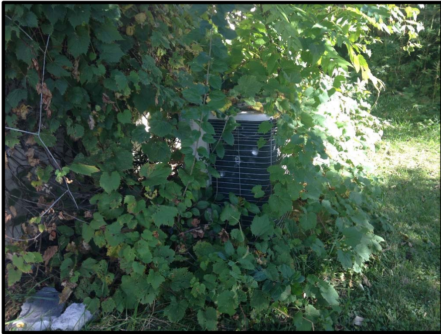
VIEW OF THE AIR CONDITIONING UNIT LOCATED ON THE SOUTHERN SIDE OF THE SUBJECT BUILDING
