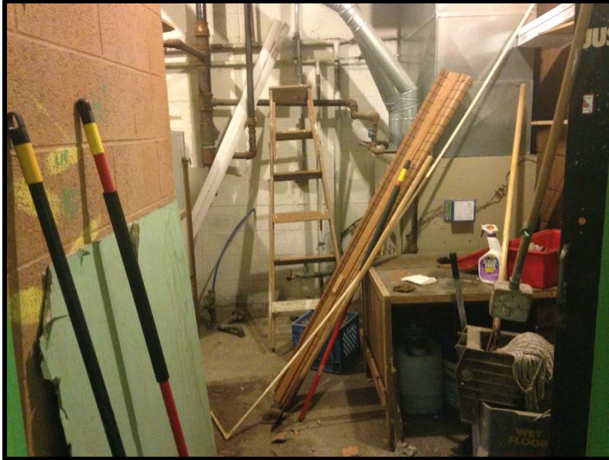
VIEW OF THE SUBJECT PROPERTY BOILER ROOM
