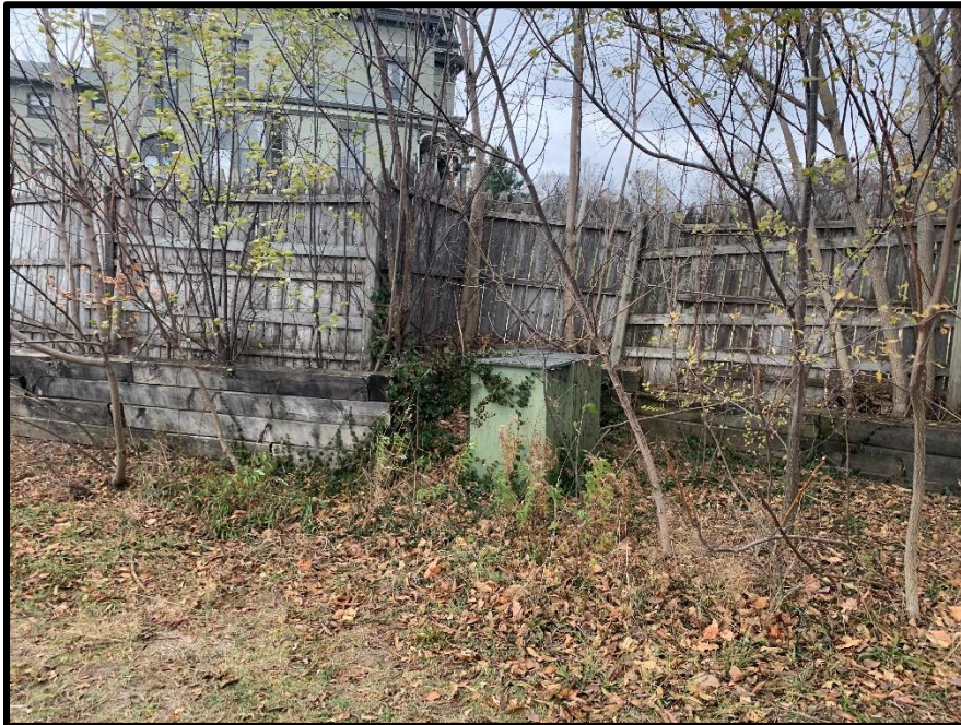
APPARENT TRANSFORMER, NORTH-CENTRAL PORTION OF SUBJECT PROPERTY
