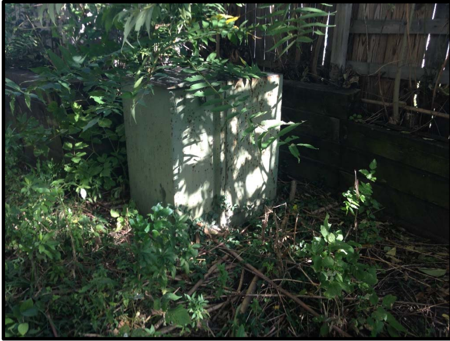
VIEW OF THE PAD MOUNTED TRANSFORMER LOCATED ON THE EASTERN SIDE OF THE SUBJECT BUILDING
