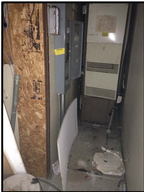
VIEW OF A THE MECHANICAL ROOM LOCATED ABOVE THE SUBJECT BUILDING GARAGE
