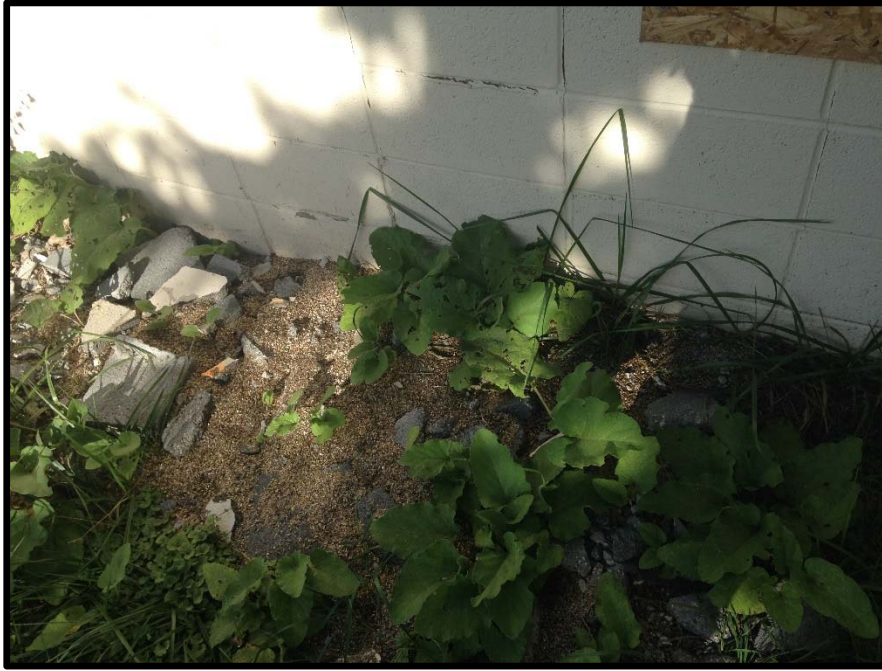
VIEW OF DAMAGED BUILDING MATERIALS LOCATED ON THE SOUTHERN EXTERIOR OF THE SUBJECT BUILDING
