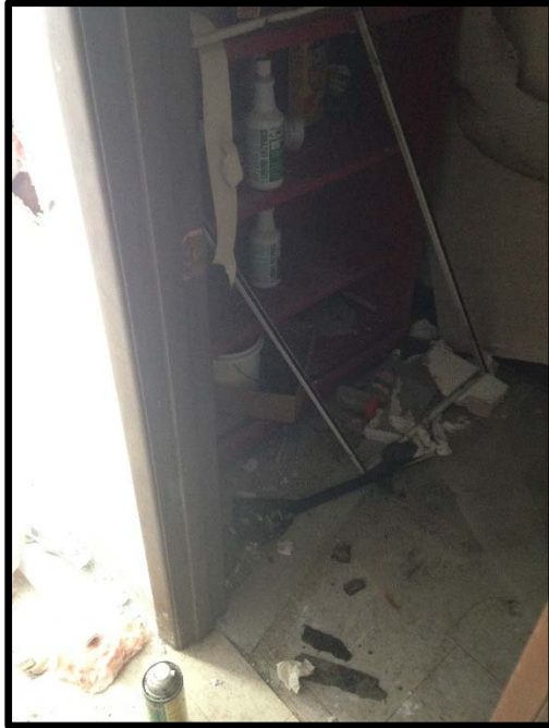
VIEW OF THE CHEMICAL STORAGE AREA WITHIN THE OFFICES ABOVE THE SUBJECT BUILDING GARAGE
