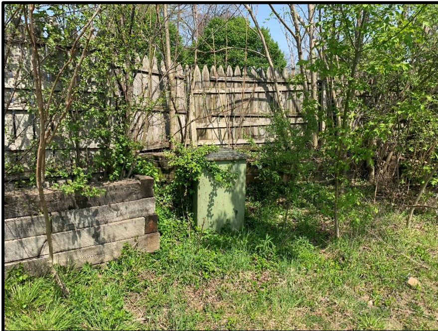
APPARENT TRANSFORMER, NORTH-CENTRAL PORTION OF SUBJECT PROPERTY
