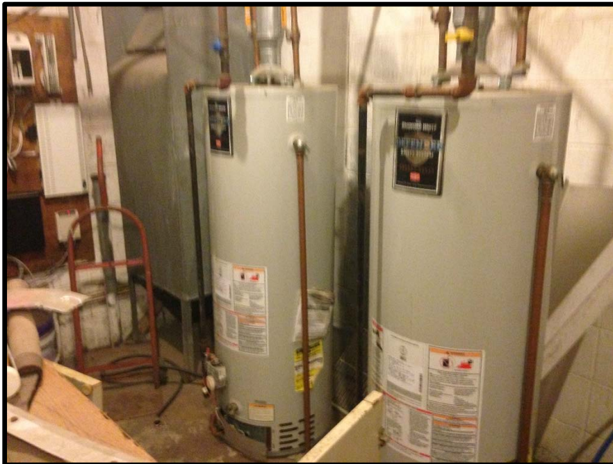
VIEW OF THE SUBJECT BUILDING BOILER ROOM
